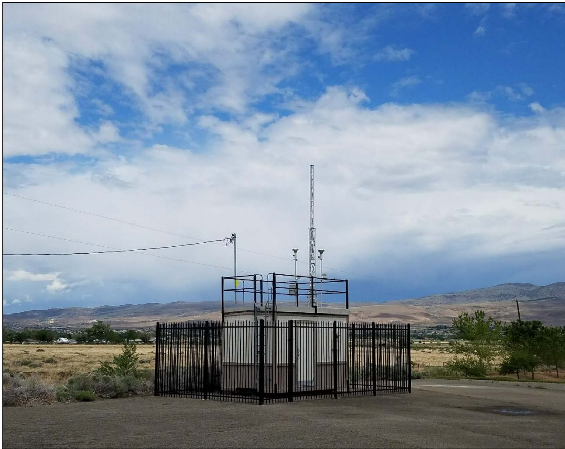
Figure 14 Spanish Springs Monitoring Station
