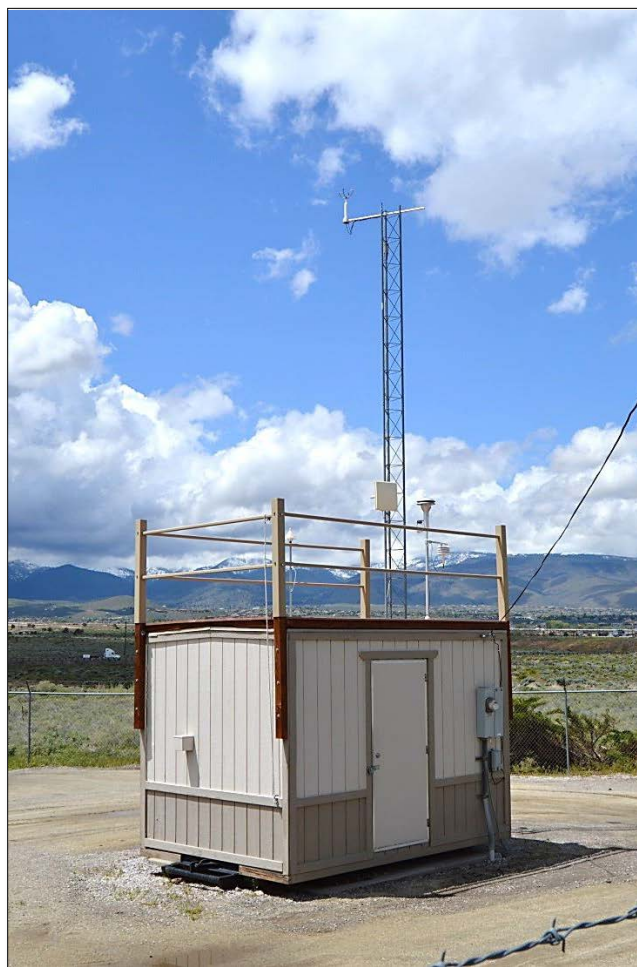
Figure 18 Toll Monitoring Station
